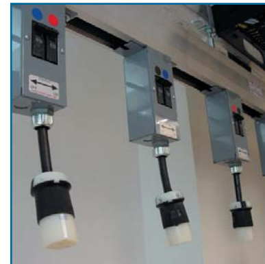
Each power module is circuit protected with circuit breakers or fuses right at point-of-use.
